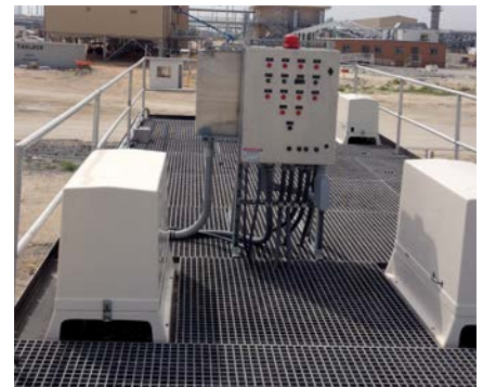
Electrical Control Console
