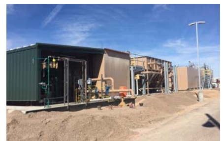
Complex treatment system servicing industry needs.
