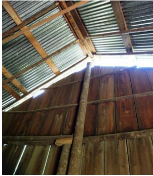
Figure 4a. Gap at ridge.
