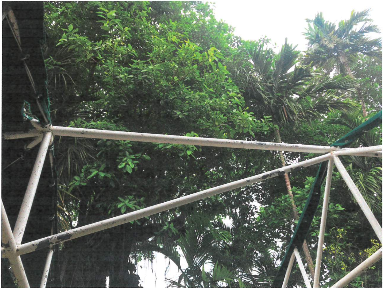
View from within the carport where you can see how all the tree branches have propelled and ripped carport.
