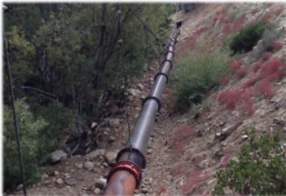
Figure 7.6: Suspended Pipe (Whitewater Flume System)
