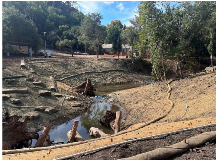
Figure 2 - Post-project conditions upstream of pedestrian bridge, featuring placed log structures and constructed riffles.
