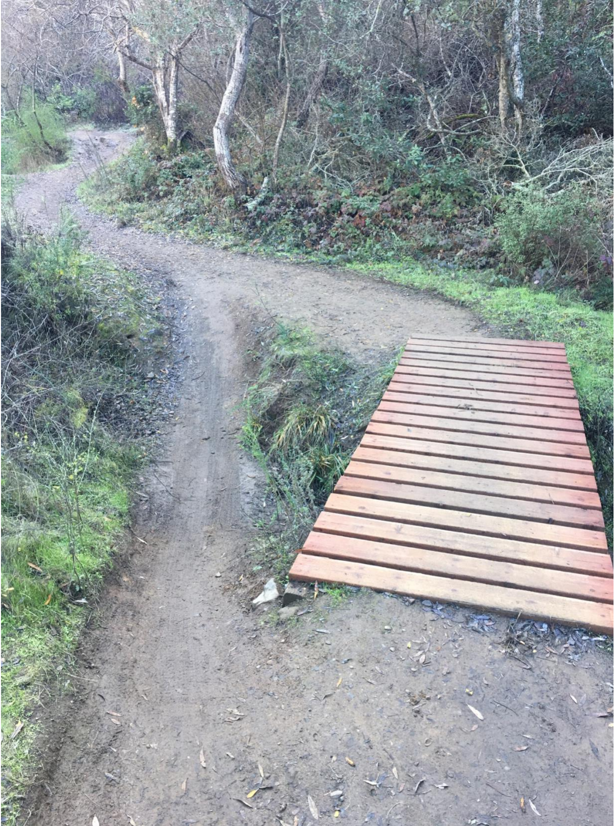
Figure 12. Dry crossing being bypassed by trail users on the Canyon Creek Trail.
