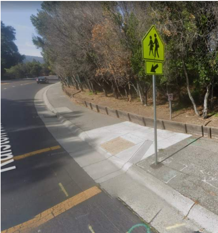
"Before" non-ADA compliant curb ramp transition to AC path at Chula Vista
