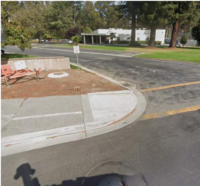
"Before" non-ADA compliant curb ramp transition to AC path
