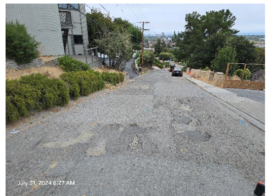
Figure 1 - Typical roadway conditions on project segment prior to reconstruction.
