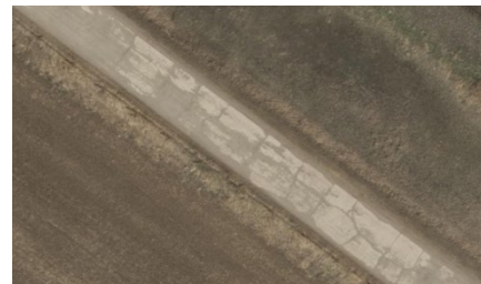
Figure 1: Crumbling Pavement of Red Wing Dr.
