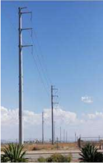
Typical transmission line on steel monopole up to 130 feet
