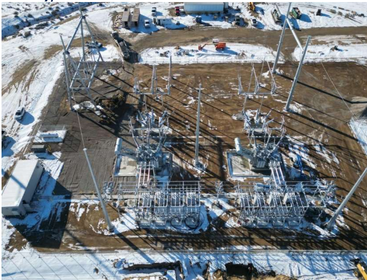
Typical substation with control enclosure. Lightning masts up to 27 feet 4 inches
