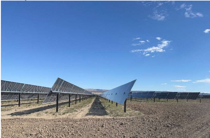
Solar PV Modules on trackers, two panels in portrait typically up to 19 feet
