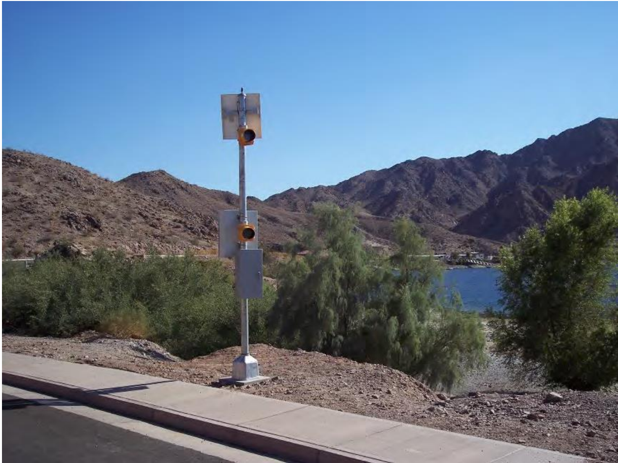
Figure 1. Automatic Roadway Flasher Pole
