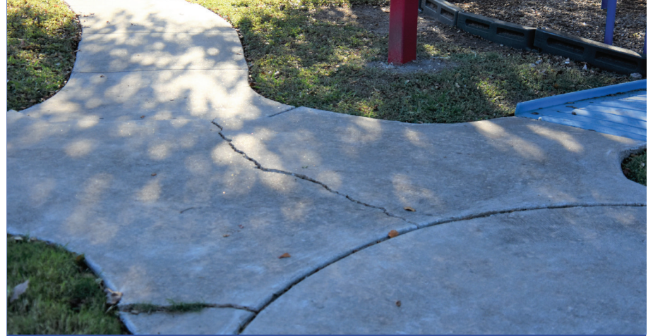
The pathways in Stoneridge Park need repairs to cracked concrete.
