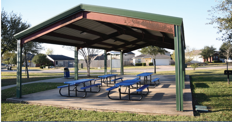
The pavilion at Green Meadows Park needs repainting and repair to damaged columns.
