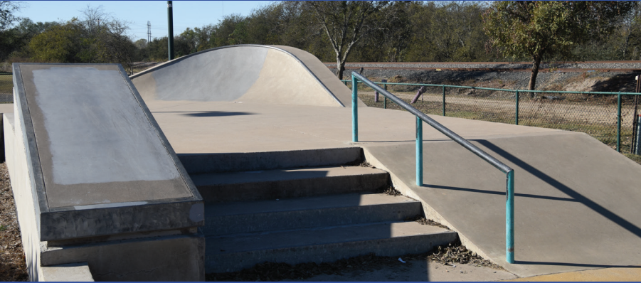
All rails and painted surfaces are in need of a new coat of paint in the skatepark.
