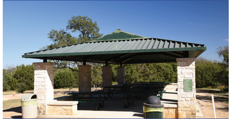
The pavilion roof at Stagecoach Park needs to be repainted.
