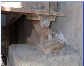
Bearing movement at Abutment 6
