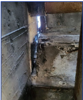
Inadequate joint seal at Abutment 6
