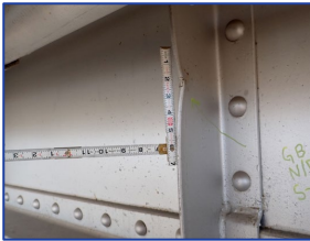
One-inch bend in stiffener
