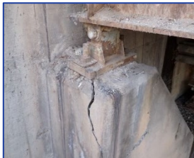
Bearing pedestal crack
