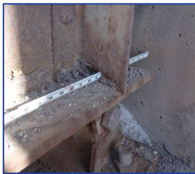
Hole in girder stiffener
