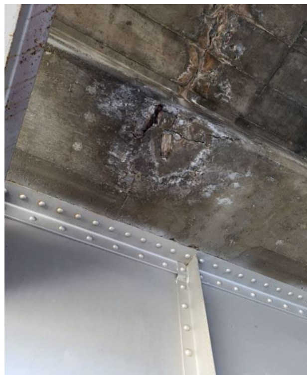
Figure 12. Deck Concrete Spall with Exposed Rebar
