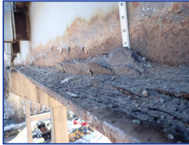
Considerable girder corrosion
