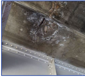
Deck concrete spall with exposed rebar
