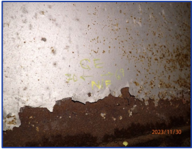
Failure of protective coating
