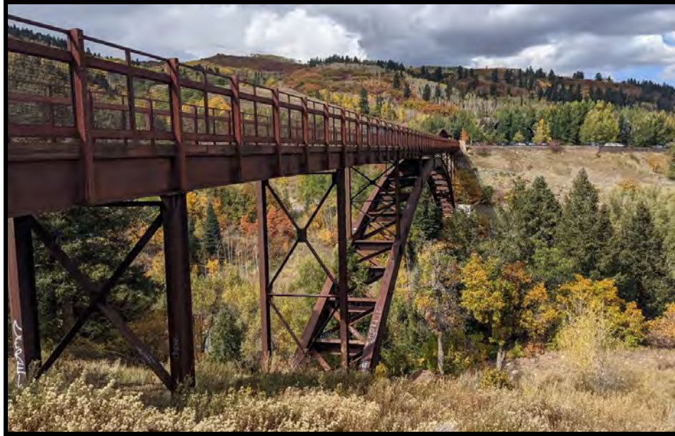
Figure 4-4: Terral Wade Bridge (Tiehack Nordic Bridge, 605 LF) Aspen, Colorado. Weathering Steel Deck Arch
