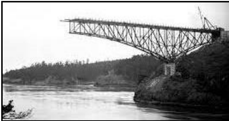
Figure 4-10: Deception Pass Bridge during Construction, Whidbey Island, Washington. (Imagery Courtesy of WSDOT)
