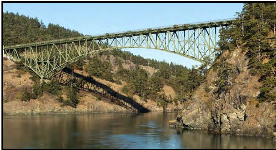
Figure 4-8: Deception Pass Bridge Whidbey Island, Washington. Steel Deck Truss (Imagery Courtesy of Frank Schulenburg)
