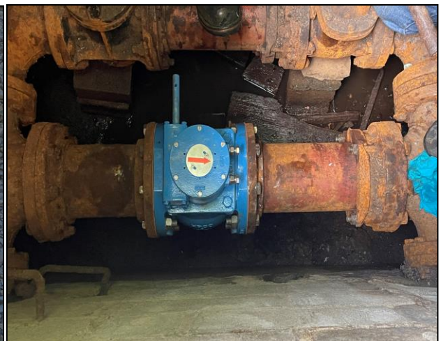
Cargill Reservoir Control Valve
