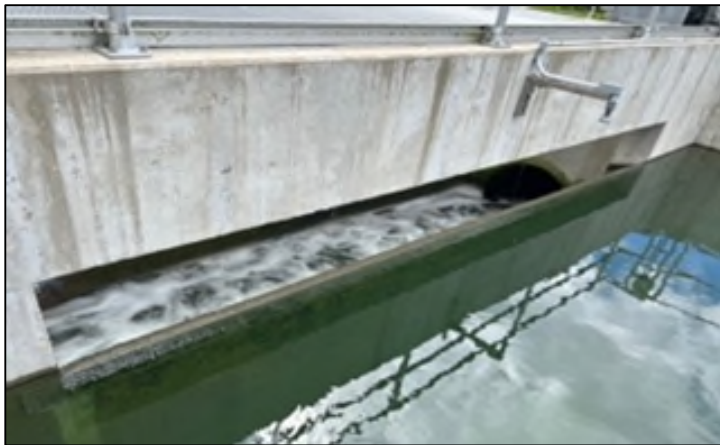
Chlorine Contact Tank for Wastewater Disinfection
