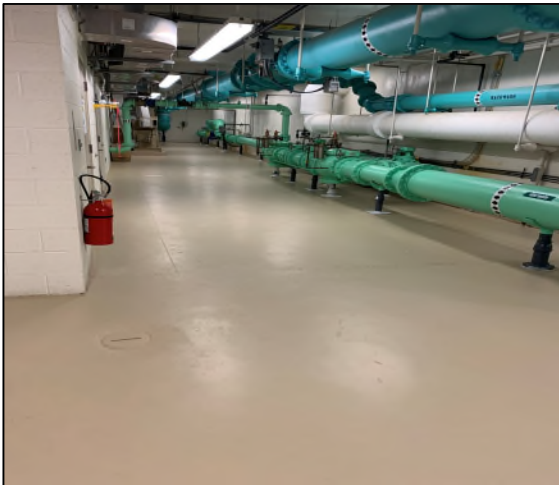
Pipe Gallery at Water Treatment Plant
