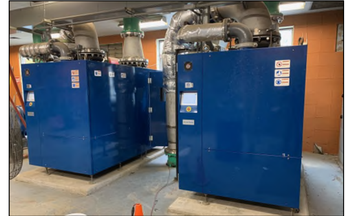
Aeration Blowers to be Replaced in 2026 Transition to Smaller Units
