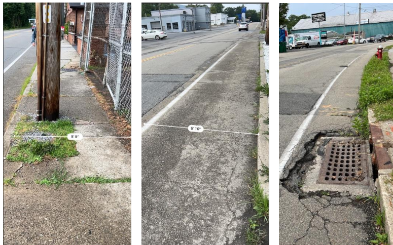
Figure 9. Sidewalk obstructions, narrow shoulder, and storm grates make difficult conditions for pedestrians and cyclists along Fishkill Avenue
