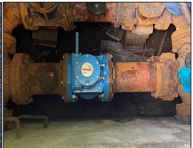
Cargill Reservoir Control Valve
