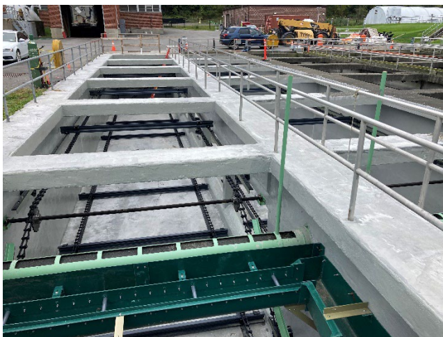
Primary Setting Tanks
