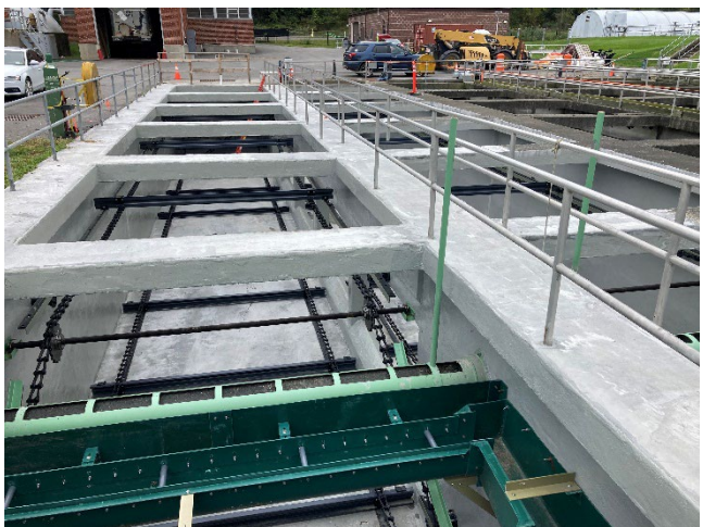
Primary Setting Tanks
