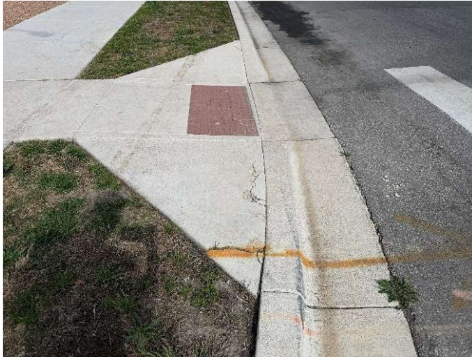
ADA ramp with cracks present.
