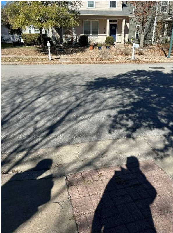
ADA ramp on Negley does not connect to a usable path.
