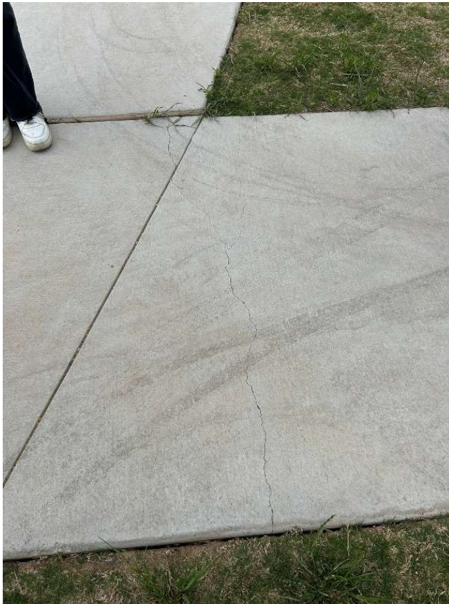
Cracked sidewalk panel on Ramage school property.
