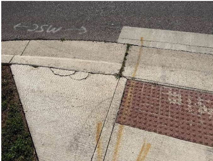
ADA ramp with cracks present and tactile indicators in poor condition.
