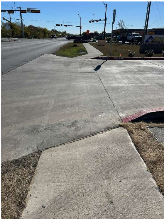
Sidewalk is not continuous; driveway interruptions
