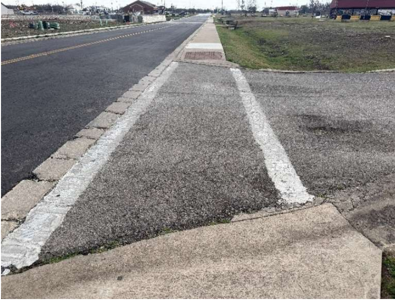
(Top & Bottom) Driveway interruption located at parking lot to Gregg-Clarke Park, curb ramp in poor condition.
