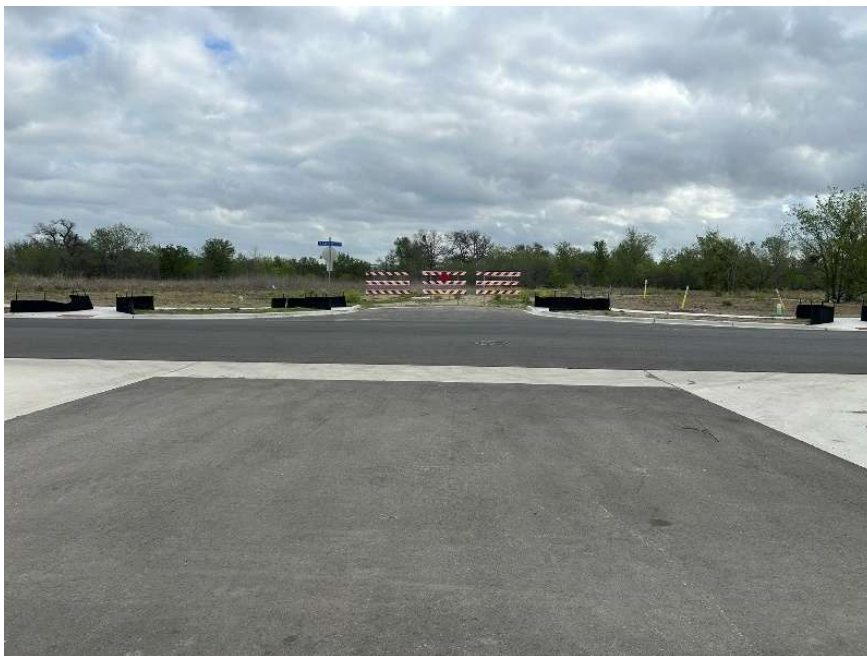
Intersection lacks crosswalk markings.
