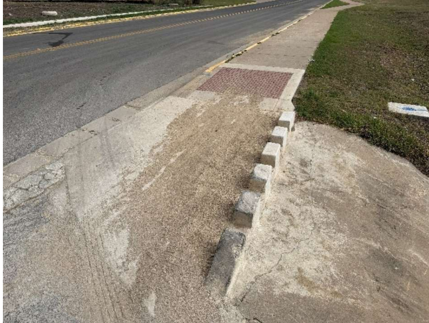
Sidewalk crosses drainage pathway and has sediment buildup.
