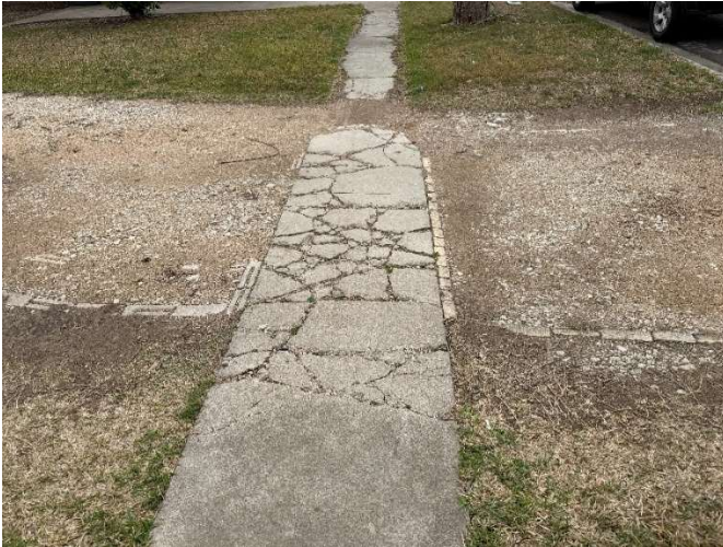
Sidewalk along Blanco Street between N Wallace and N Meyer is in very poor condition, with severe cracking.
