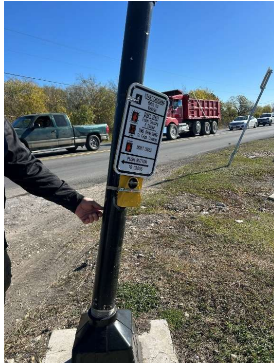
Push-to-walk mechanism not optimally placed and shows signs of damage.
