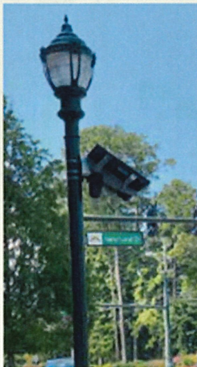
Solar & Existing Pole
