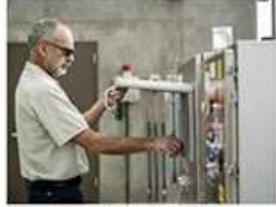
Michalak, at the control panel for the two-basin L-shaped Equipment Corporation, got a late start in the clean-water profession but has found it rewarding.
