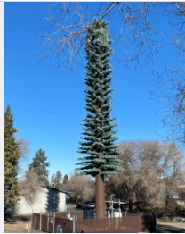
b. Monopine (Faux Tree)
