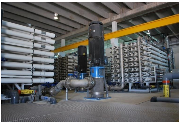
Figure C.5 RO modules (Photo credit: City of Wichita Falls)
