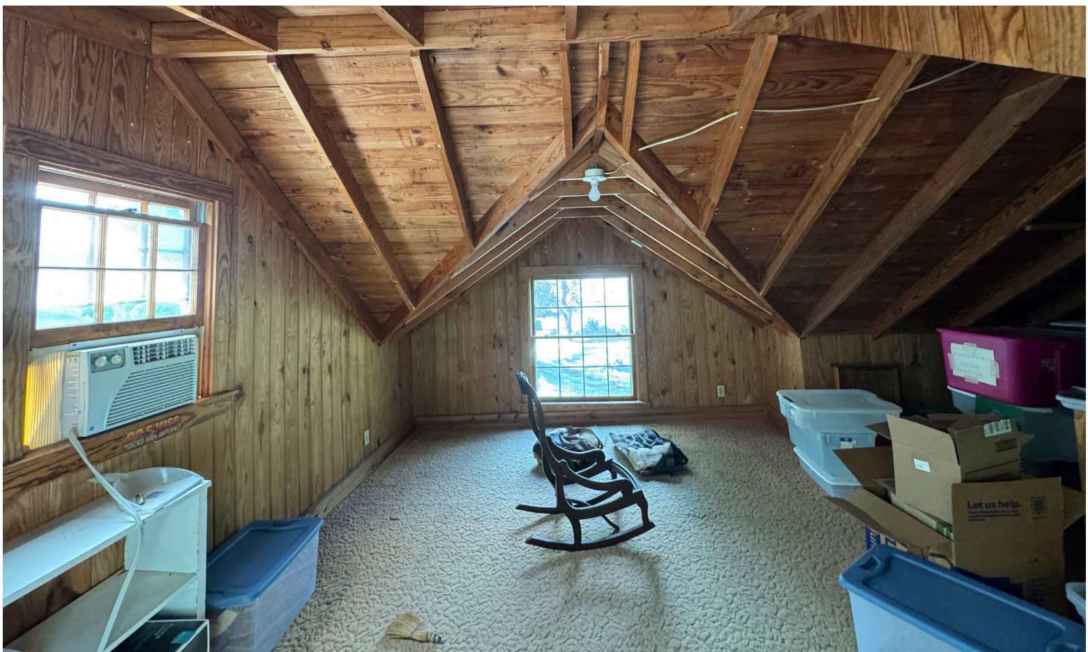
1970S NON-CODE COMPLIANT ATTIC / BEDROOM TO BE REMOVED
