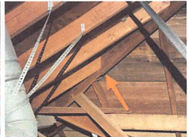
Unsupported hip rafter splice
