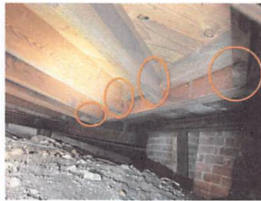
Missing joist hangers
