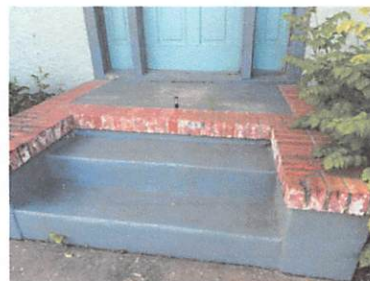
riser variance exceeds 3/8"
