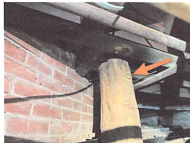
pier tilted and not supporting beam near fireplace
