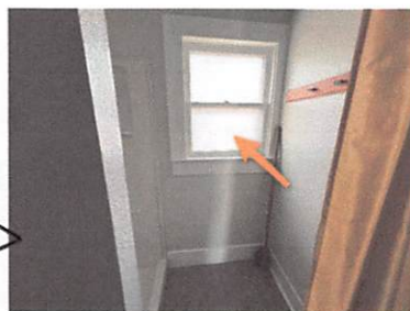
Missing tempered glass next to shower in bathroom
