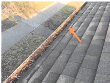
Clear debris from gutters
