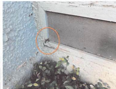
Various trim damage
