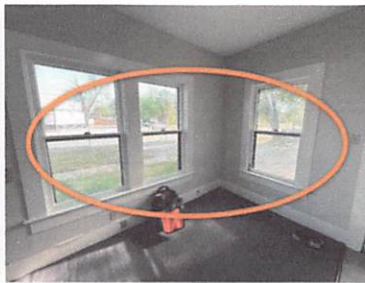
Windows appear painted shut. Living room
