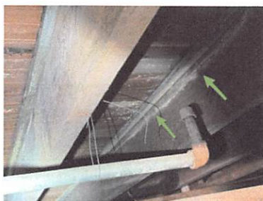
Visible fungal growth within crawl space
