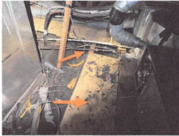
Walkway segmented and service platform less than 30 inches in front of HVAC equipment
