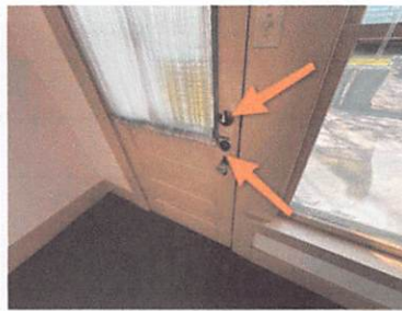
Back door. Bottom deadbolt inoperative. Top deadbolt difficult to operate
