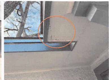
Soffit damage due to previous water penetration
