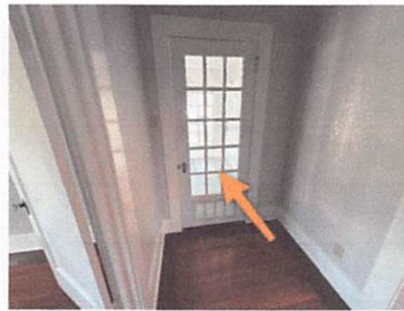
No tempered glass etching observed at right side bedroom door
