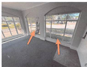
Window panes over 9 square feet missing tempered glass. Right side room
