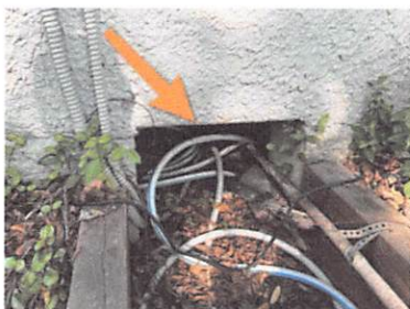
Exterior crawlspace access undersized (18" x 14")
