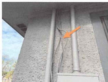
Exposed and unprotected wiring
