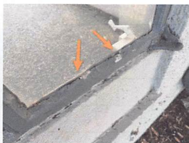
poor window glazing compound
