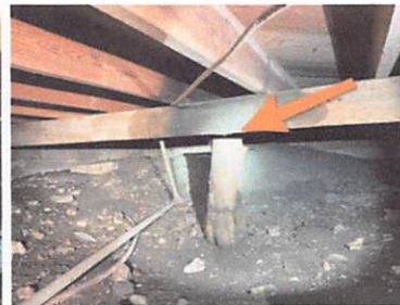
pier no longer supporting beam
