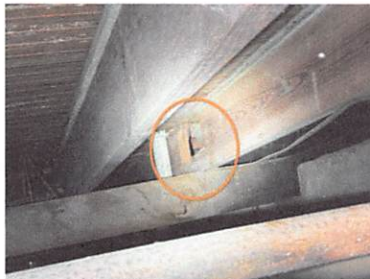
Improper joist notch and bearing under shower
