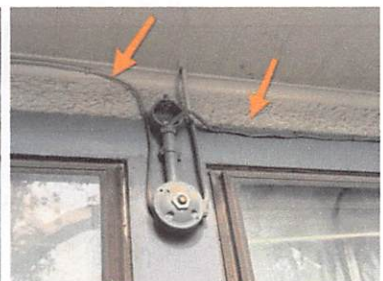
Exposed and unprotected wiring
