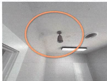
Back bedroom. Appears to be below HVAC unit in attic
