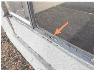
poor window glazing compound
