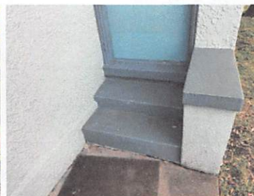
riser variance exceeds 3/8"
