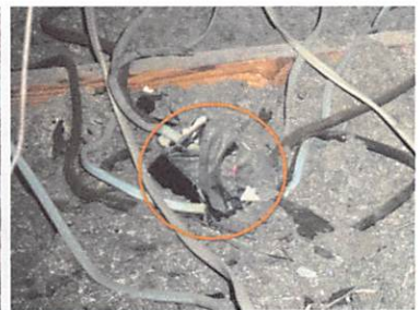
Exposed wiring connections in attic
