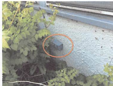
Missing appropriate wet location cover
