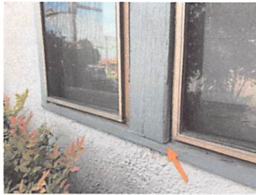
Loose and deteriorating trim
