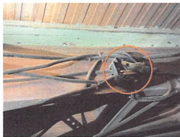
Exposed wiring connections within crawlspace
