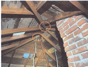
Unsupported hip rafter ends
