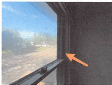
Damaged lift support. Back left side room.
