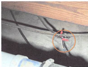
Exposed wiring connections within crawlspace
