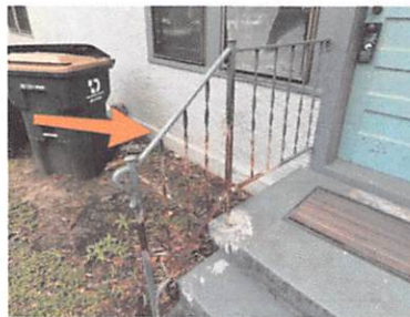
Rear - substantially loose handrail
