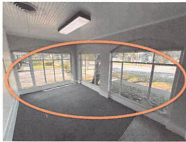
Windows appear to be painted shut. Back right side room.
