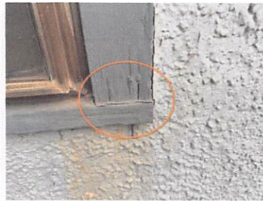
Wood rot and potential water entry points
