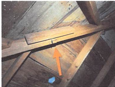
Unsupported hip rafter splice
