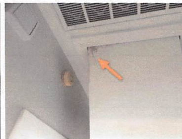
Attic stair unit
