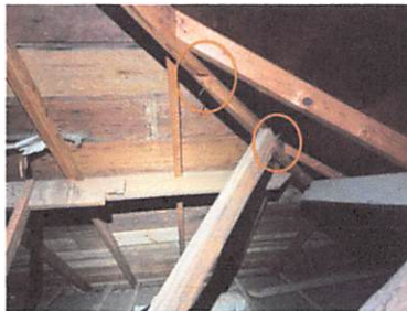
Previous splice support detached
