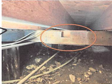
notched and subsequently repaired beam
