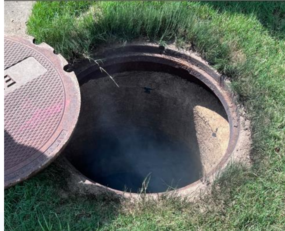
Figure: Smoke coming from fault from underground electrical system in Sun City.
