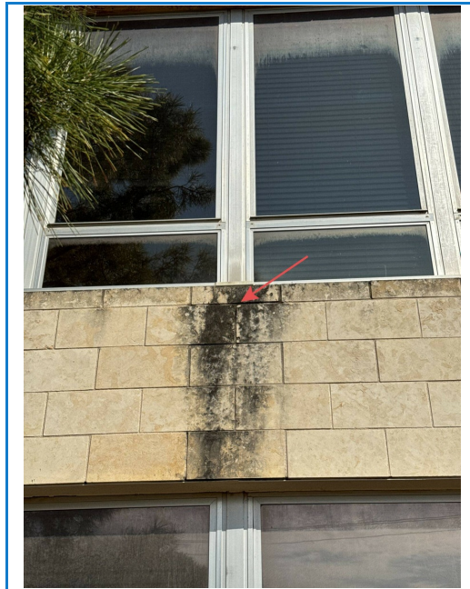
8. 02/12/2026 04:09 PM Asphalt staining directly below location of previous asphalt flowing from roof edge metal
