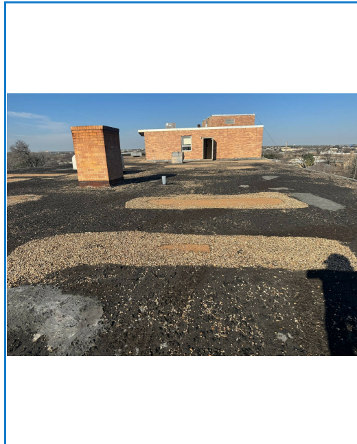
2. 02/12/2026 02:24 PM East roof area, note missing gravel and extensive repair areas
