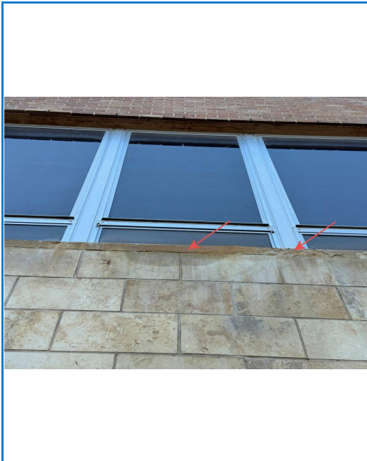
11. 02/12/2026 03:48 PM Active water penetration from roof staining and deteriorating exterior cladding on the Northwest elevation
