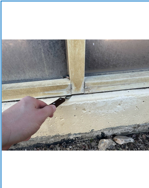
17. 02/12/2026 03:48 PM Sealant and backer rod was not evident around the perimeter of the storefront system
