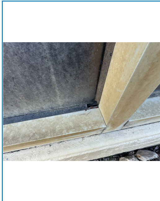
18. 02/12/2026 03:48 PM Shrinkage of the existing glazing gaskets on the storefront system
