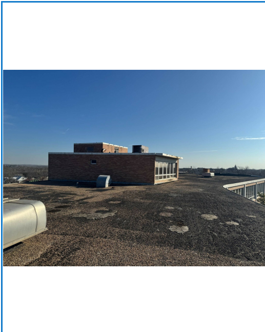
1. 02/12/2026 02:33 PM West roof area, note missing gravel and exposed asphalt
