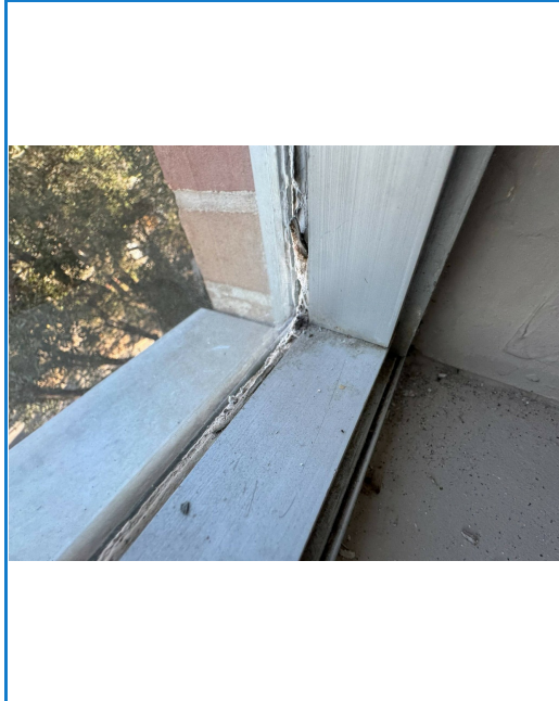
11. 02/12/2026 02:52 PM Typical failed glazing sealants around single pane glass
