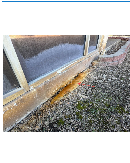
10. 02/12/2026 03:48 PM Extensive active dripping with mineral deposits from roofing system concentrated on the Northwest Elevation
