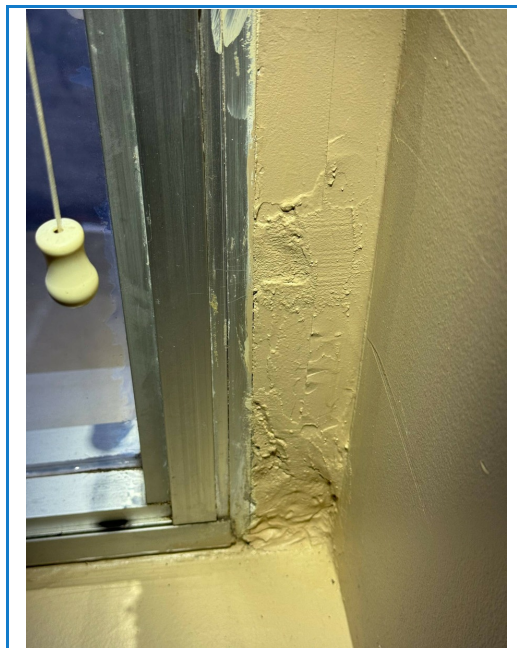
5. 02/12/2026 03:11 PM Typical interior water damage observed around the glazing systems
