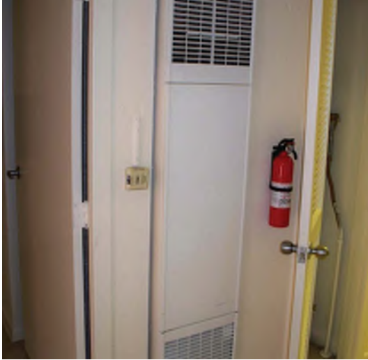
Outdated self-contained gas furnace and thermostat
