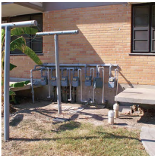
gas meters and service piping running into crawl space area. Note PVC cleanouts for sewer lines and abandoned water meter boxes in same area.
