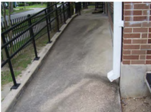
Life Safety/Accessibility: Downspout directs water onto ramp surface posing a tripping hazard.
