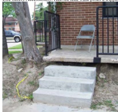
Life Safety/Accessibility: No handrail @ 3 or more risers.
