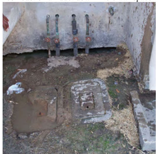
Outside water service to apartment units showing unprotected service lines, valves, and abandoned meter boxes.
