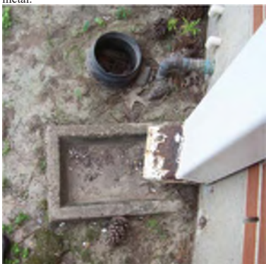
Steel downspout guards are rusted; remove and replace 35% of locations.
