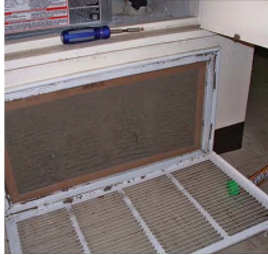
Return air filter/grill at floor
