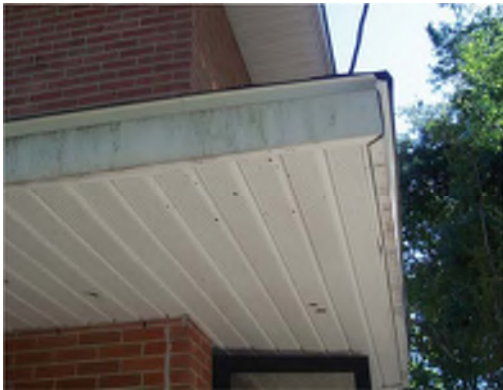
Wood warped and paint exhibits signs of water damage. Re-wrap member with metal.
