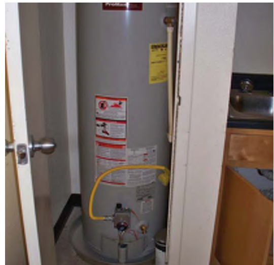
Gas water heater located in separate utility closet showing combustion air duct down into crawl space
