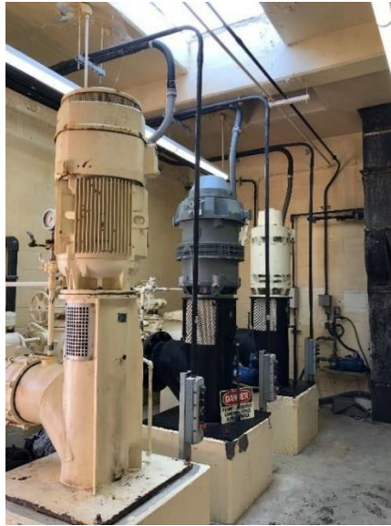
Effluent pumps 1, 2, and 3
