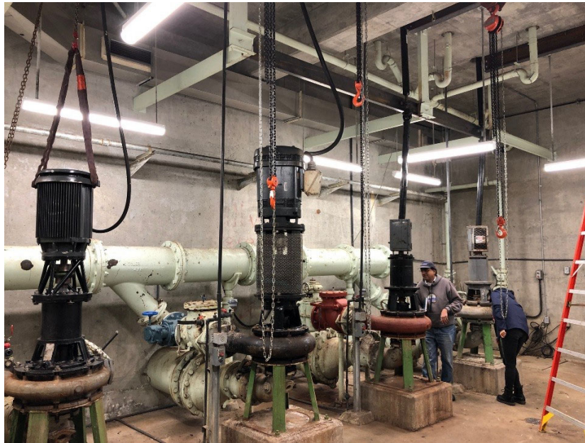
Pumps 1, 2, 3, and 4 (from left to right)
