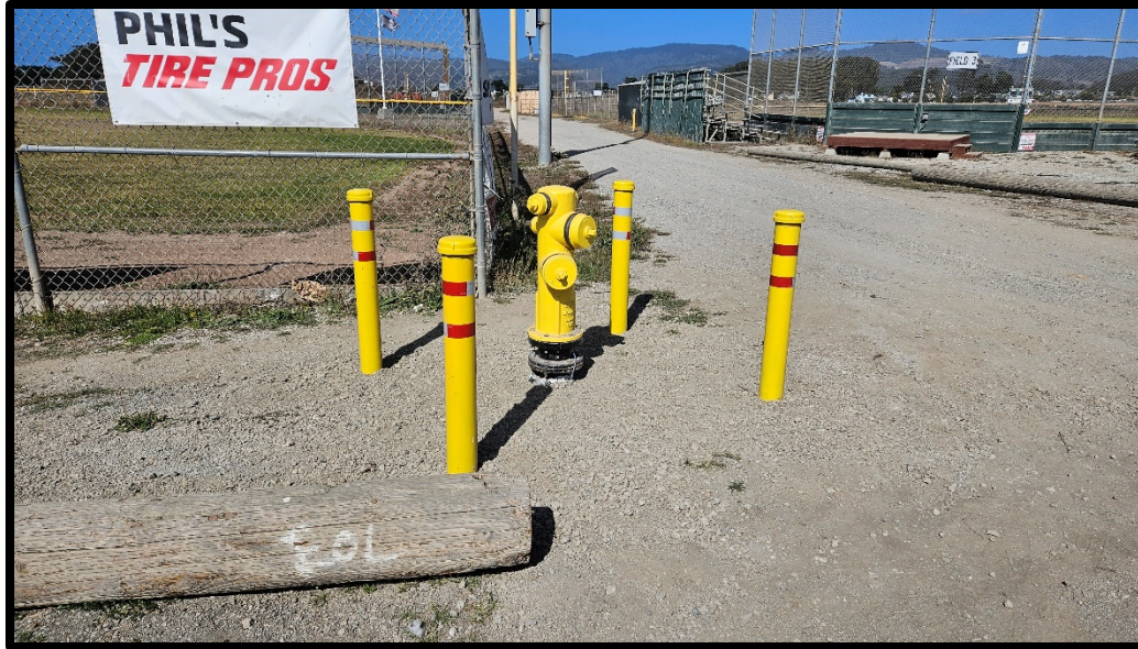
Image 2 – New Fire Hydrant at Smith Field (facing north)
