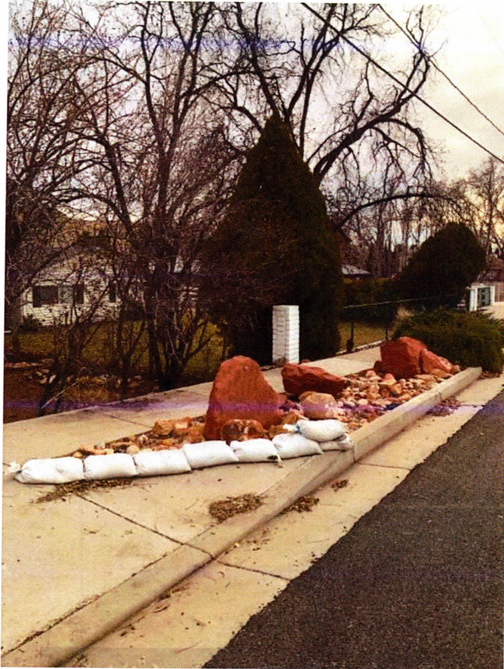
Figure 2c- Sand Bags to Prevent Overtopping of Water
