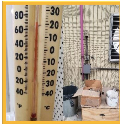
Fig 3.1: Blower Room Temperature Gauge
