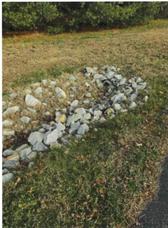
Infiltration Basin 2 inlet pipe.
