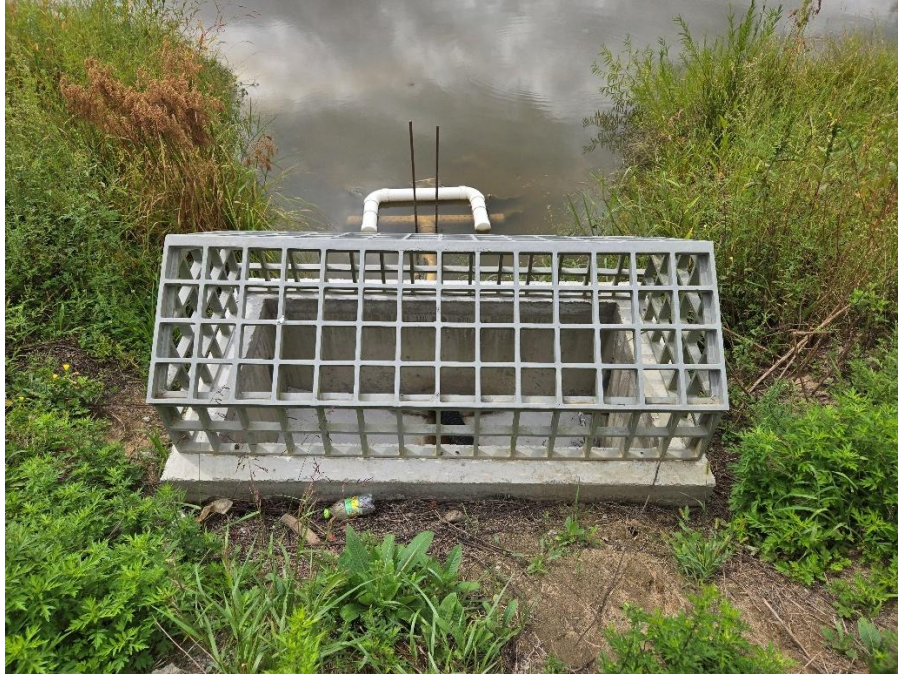
Pond 3 outlet structure with skimmer to be removed.
