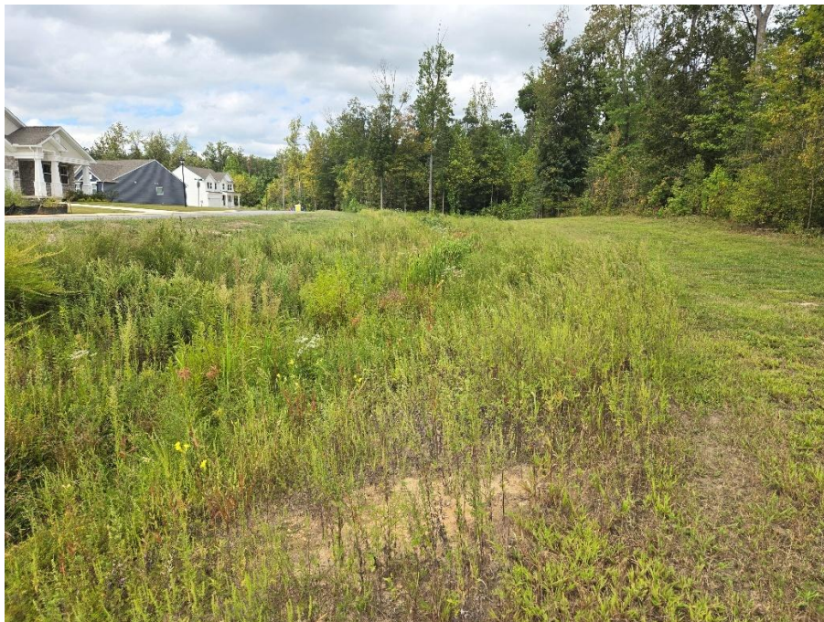
Pond 3 inlet swale with vegetation to be cut.
