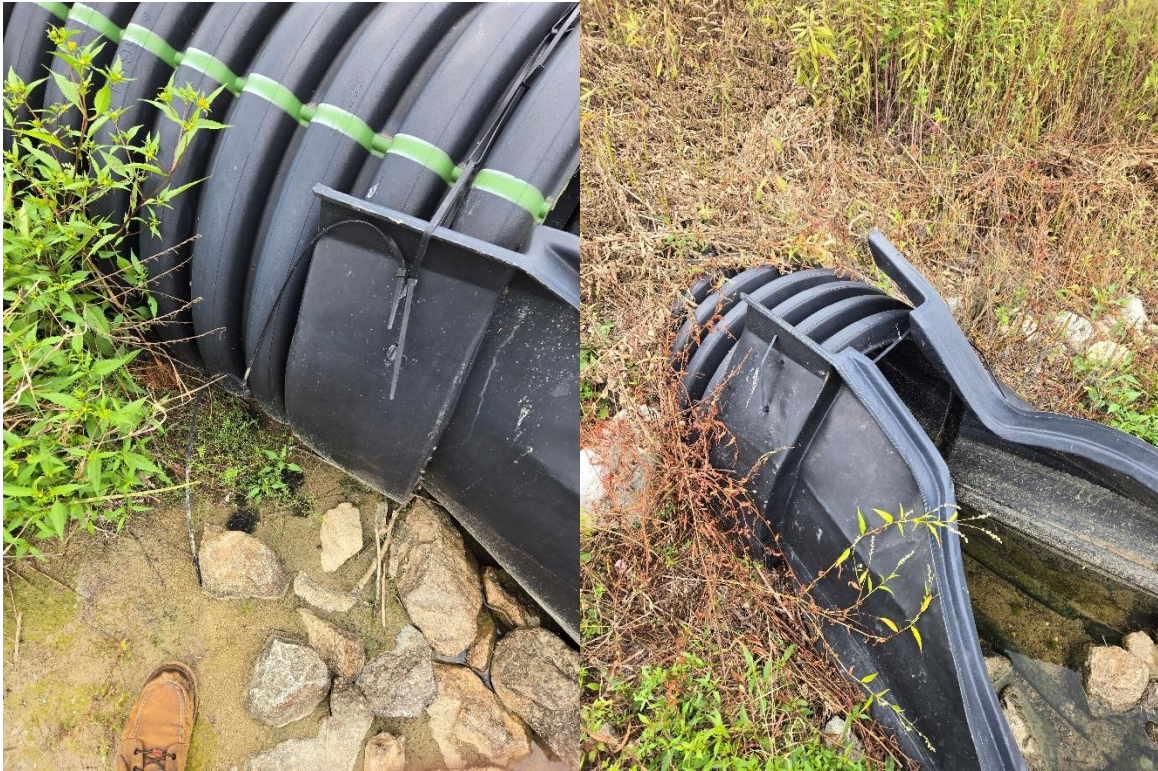
Pond 2 inlet pipes showing broken straps holding flared end sections.
