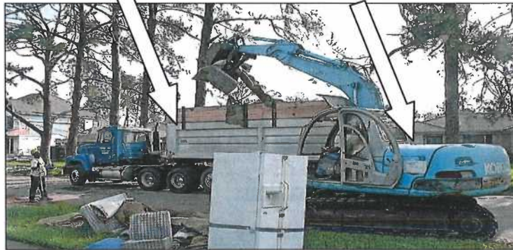
PLACARD ON EXCAVATOR
