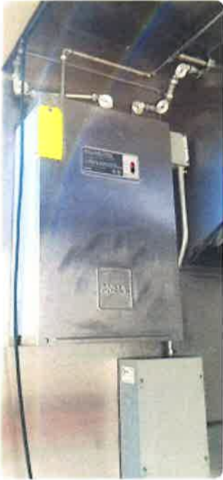
FIRE EXTINGUISHER SWITCH
