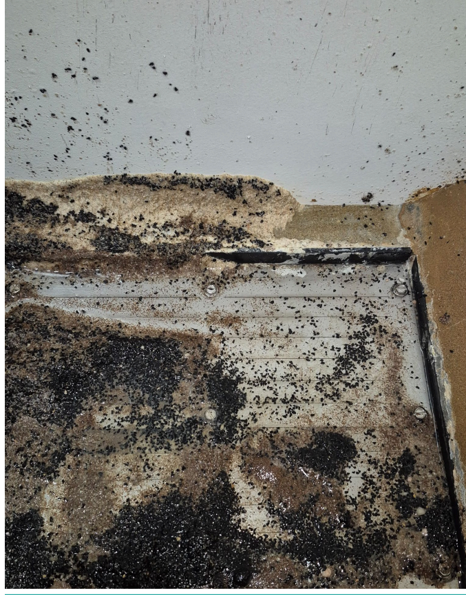
Grout not visible around internal panel area.
