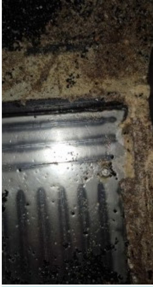
Close-up of observed condition.
