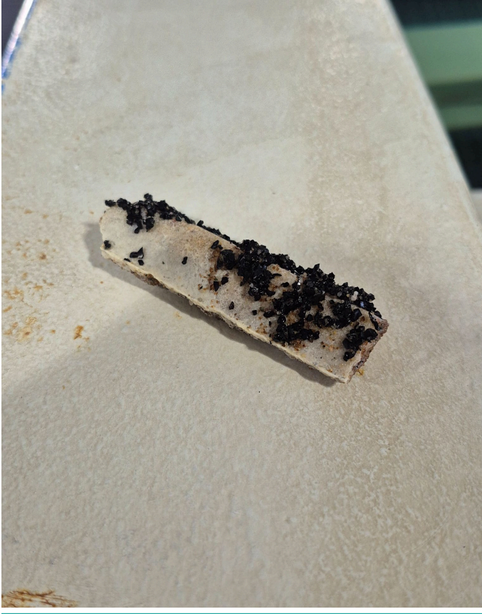
Grout Fragments coming off
