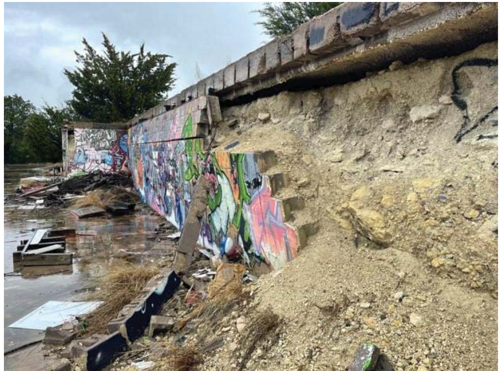
Figure 02. Partial collapse and buckling of upper wall
