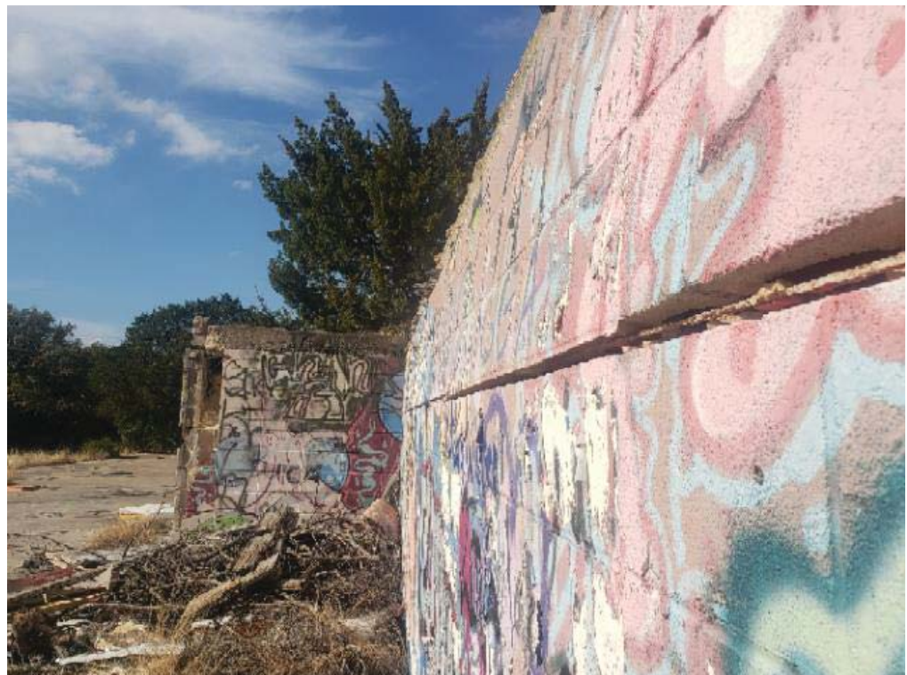
Figure 03. Faulting of upper wall
