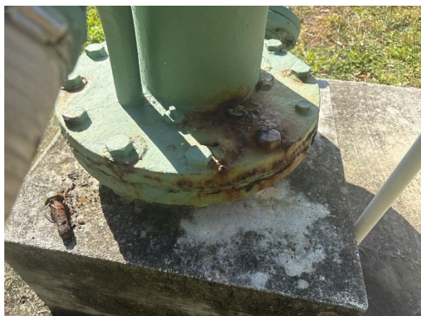
Raw Water Well No. 3
