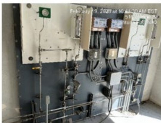
1. Anhydrous Ammonia Room
