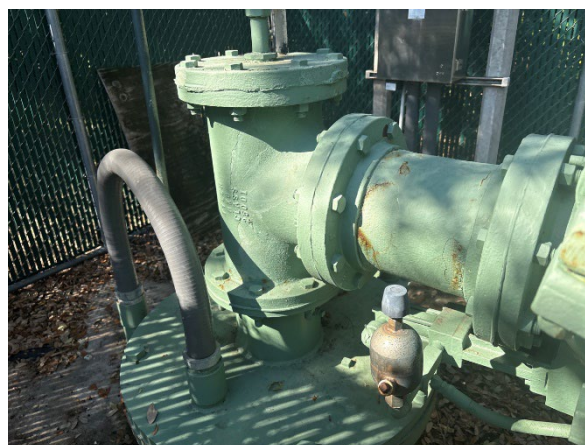
Raw Water Well No. 12
