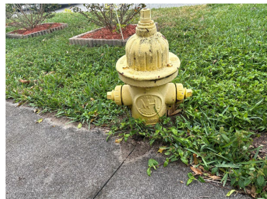
Fire Hydrant No. 297 – Below grade, rust and corrosion on surface
