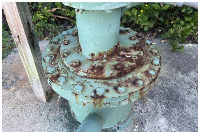
Raw Water Well No. 4
