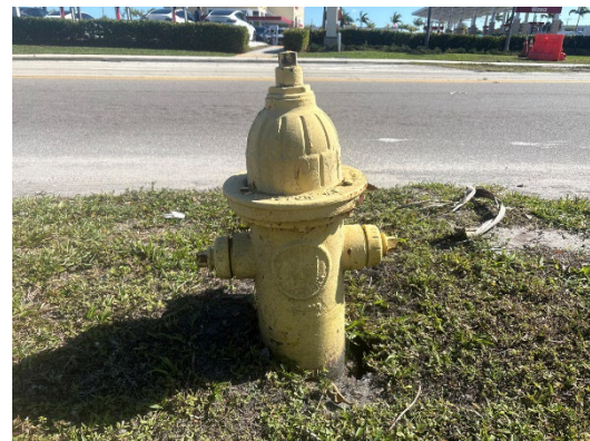
Fire Hydrant No. 240 – Below grade, rust and corrosion on surface
