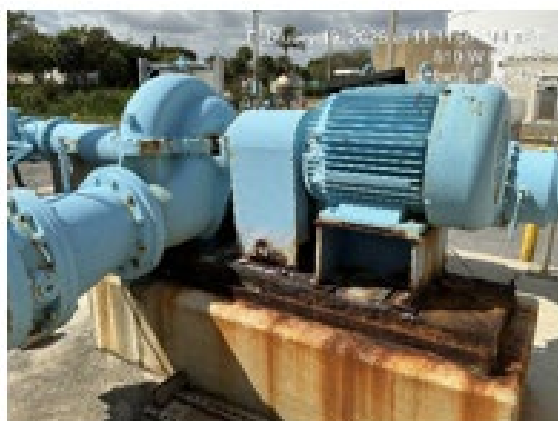
10. Filter Backwash Pumps
