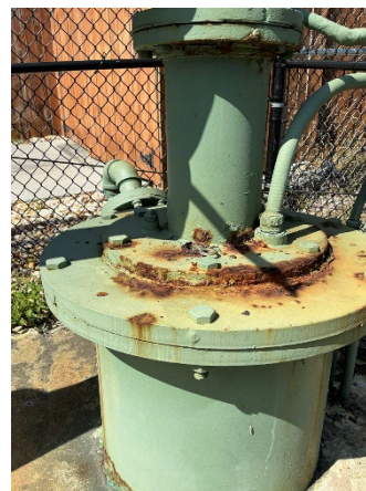
Raw Water Well No. 8
