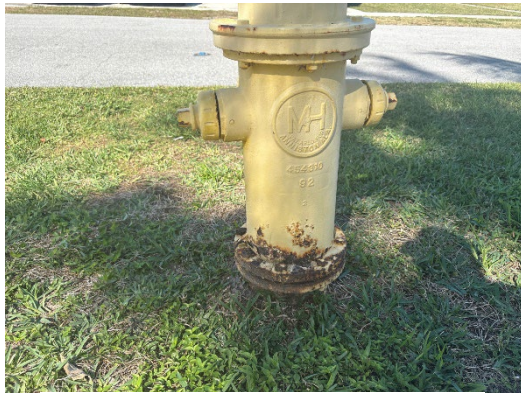
Fire Hydrant No. 130 – Bolts at base are slightly corroded
