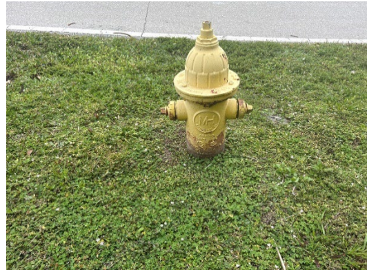
Fire Hydrant No. 82 – Below grade, no visible valve, corrosion and surface rust
