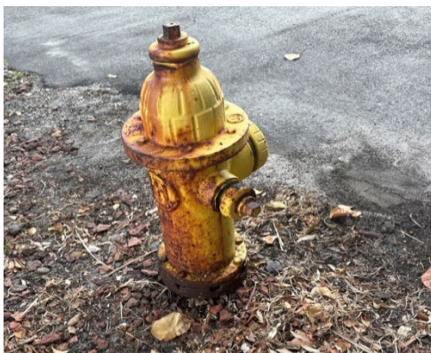
Fire Hydrant No. 268 – Significant corrosion and surface rust
