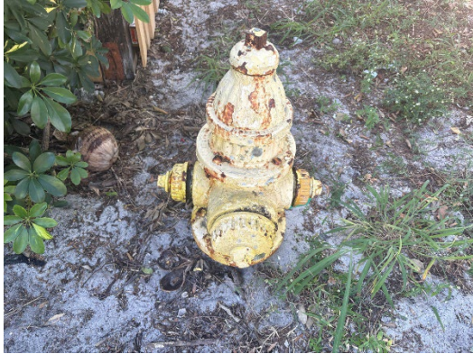
Fire Hydrant No. 41 – Below grade, significant corrosion and rusting
