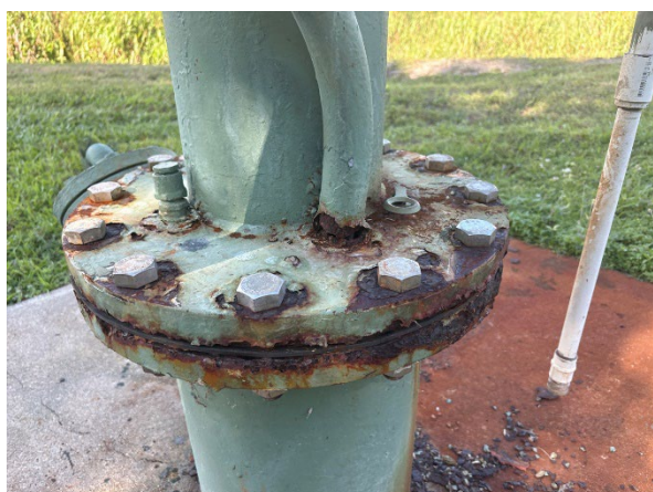
Raw Water Well No. 5
