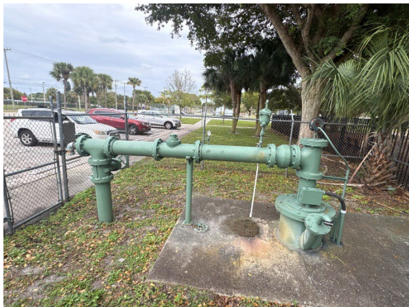
Raw Water Well No. 7
