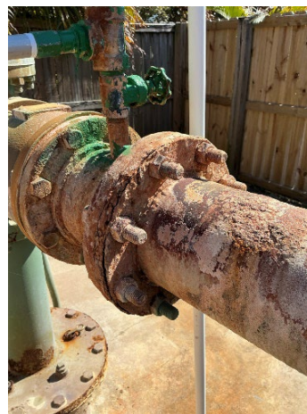
Raw Water Well No. 6
