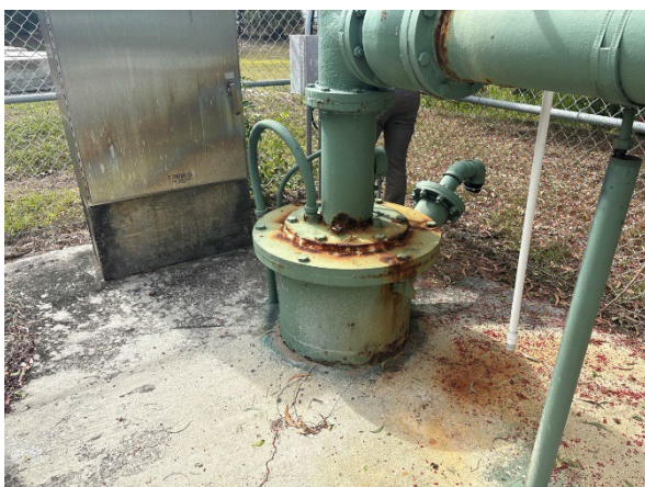
Raw Water Well No. 9
