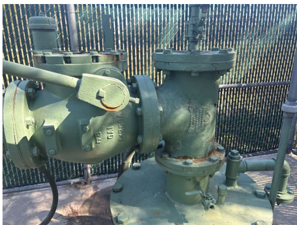
Raw Water Well No. 11
