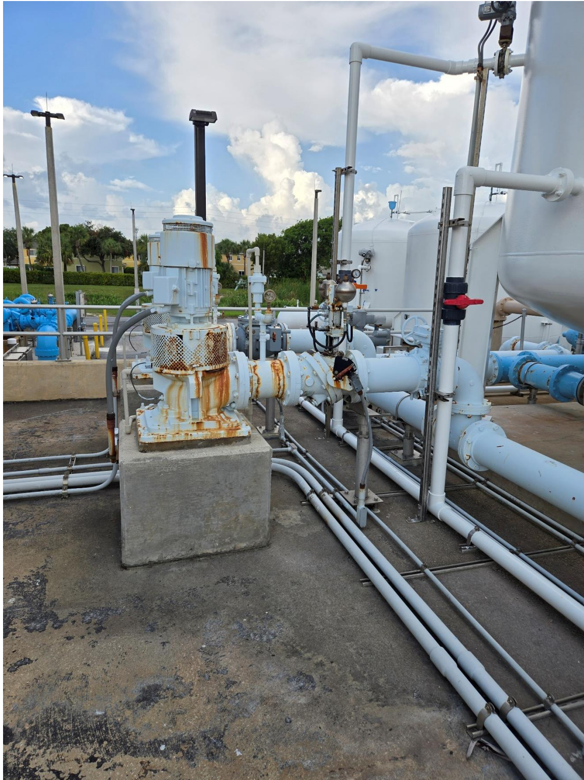
Pipes Behind Anion Exchange Unit
