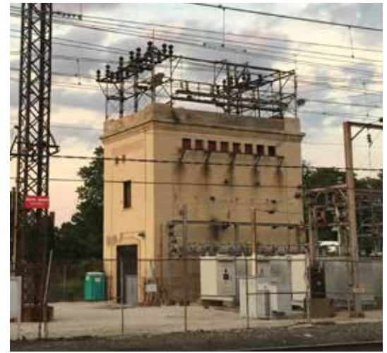
Bryn Mawr Substation
