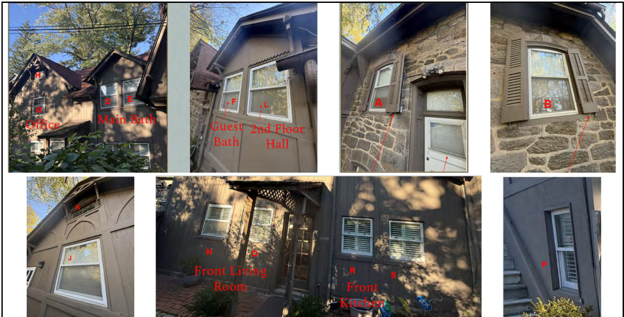
Present Non-Original Windows to be Replaced
