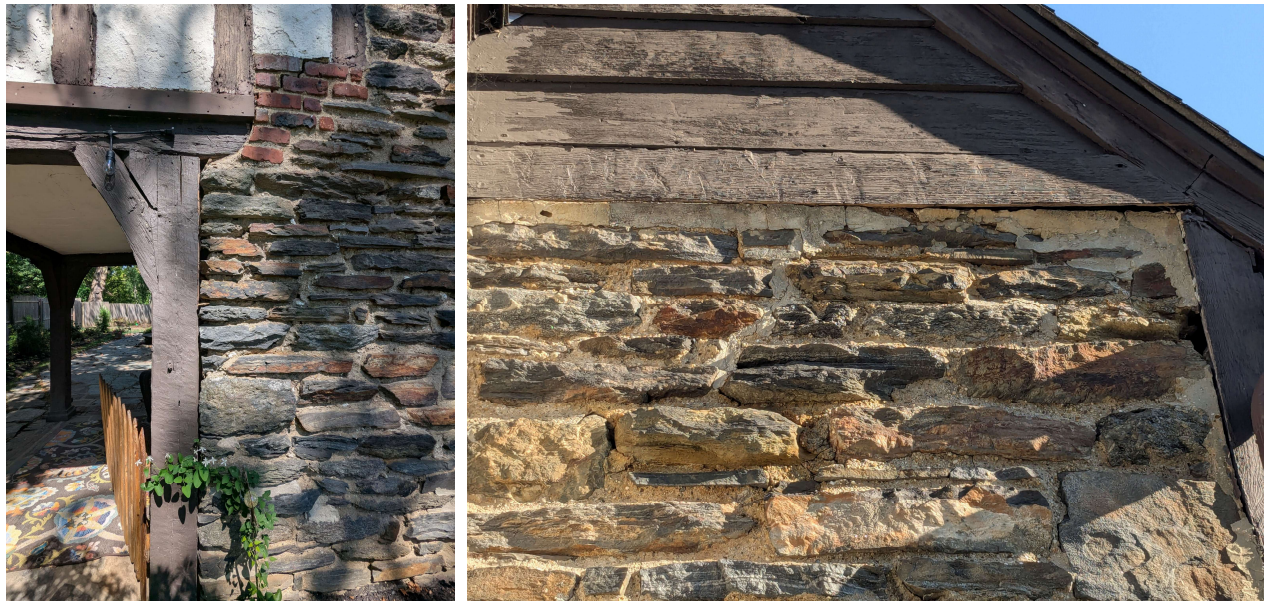
Examples of deteriorated mortar
