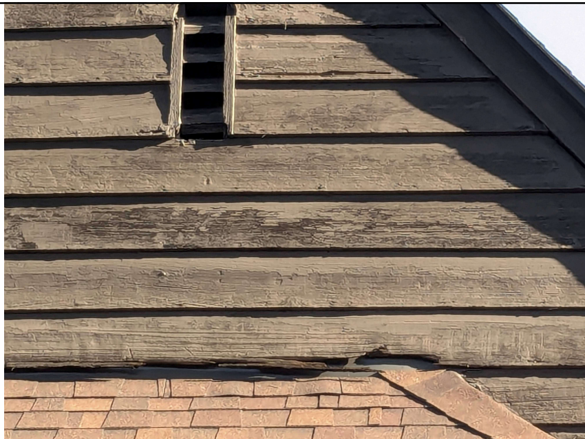
Example of deteriorated siding
