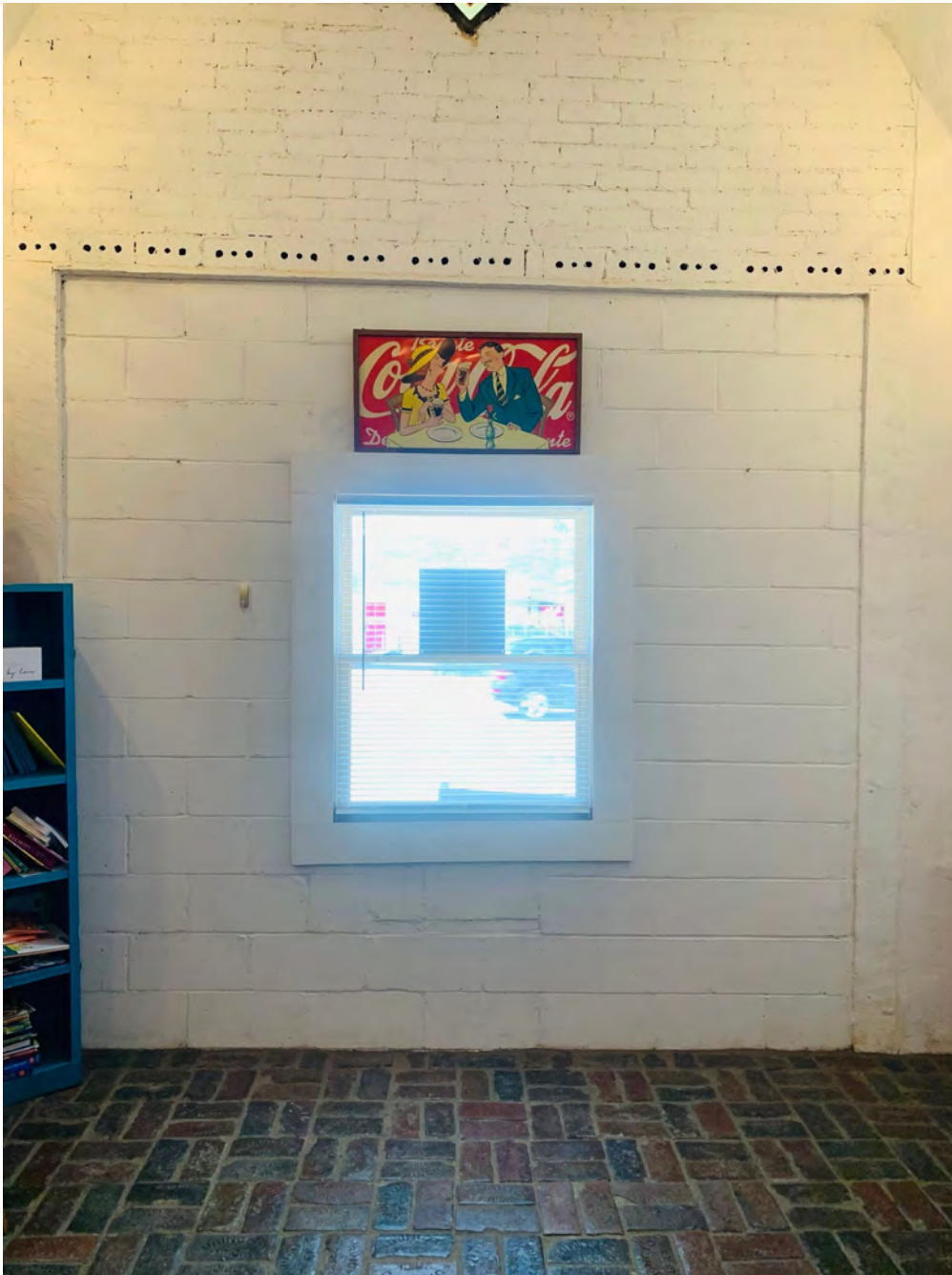
Photo 10 of 11: View from interior of enclosed service bay door opening, camera facing north.
