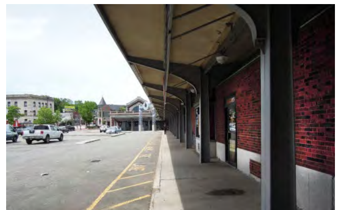
2.3-3: This recent view, comparable to the view above, shows how the 1980's brick wall interrupts the first Platform Canopy, impairing its historic integrity as a free-standing structure.
