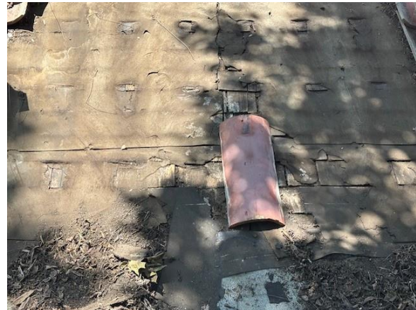
Figure F-2. Original wood shake roof exposed beneath failed tile roofing
