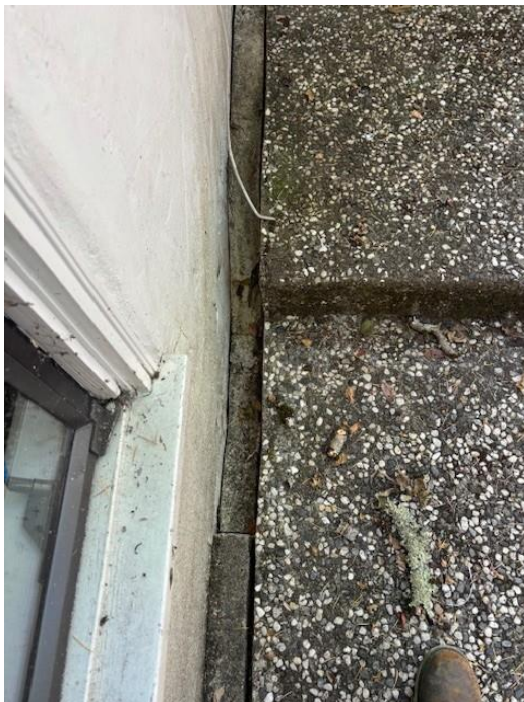
Figure F-7. Patio separation gap attributed to land movement
