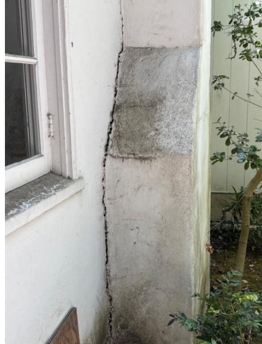
Figure F-5. Separation gap at chimney
