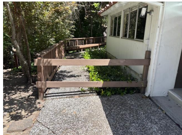
Figure F-8. Patio area closed to use due to ground movement
