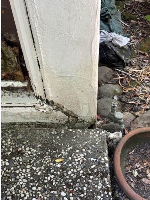
Figure F-4. Foundation cracking at exterior wall
