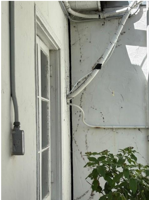
Figure F-6. Separation gap at building addition
