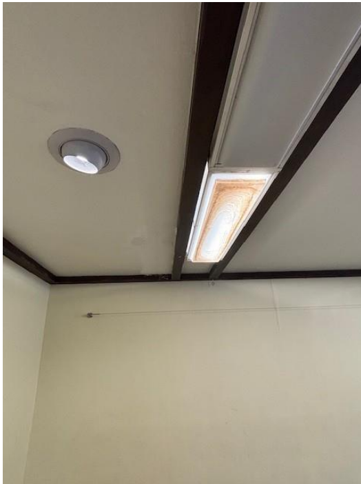
Figure F-3. Roof leak / water intrusion at interior ceiling and light fixture
