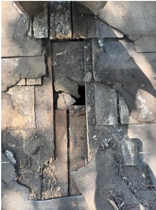
Figure F-1. Hole in deteriorated wood shake roof
